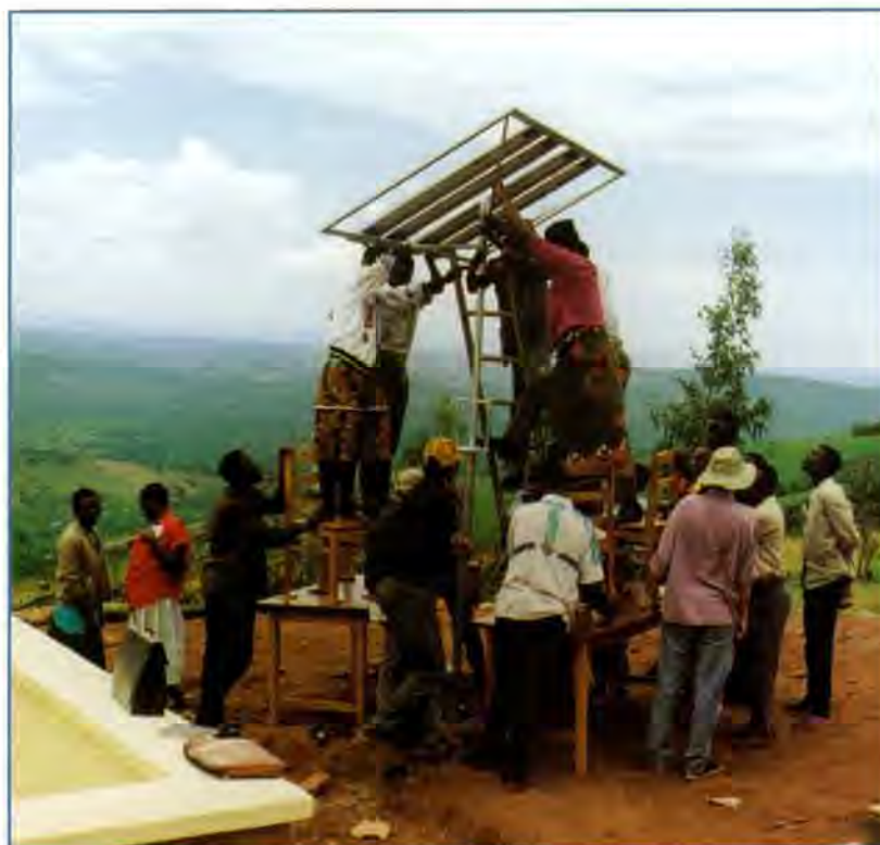
Adopting and using sustainable energies, as with these solar panels
